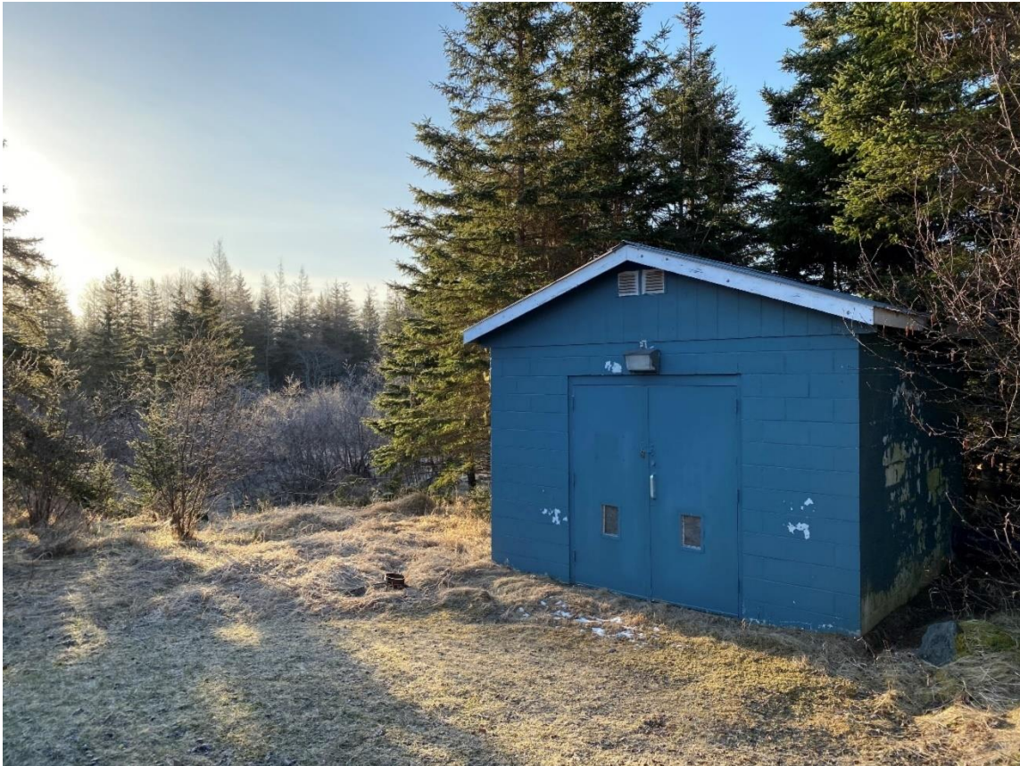
Figure 18-8: Pumping Station at Gays River
