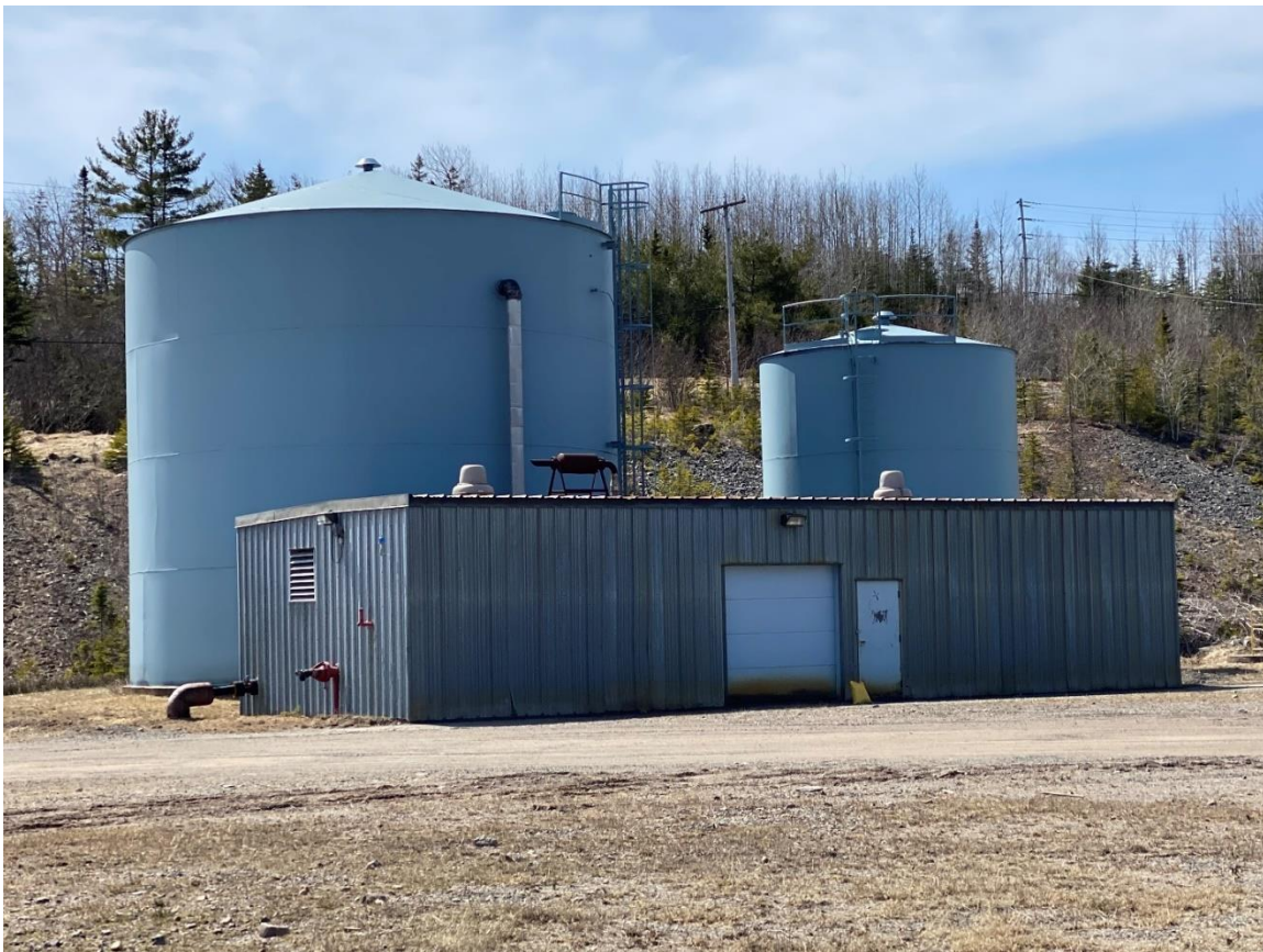
Figure 18-7: Water Treatment Plant and Water Storage
