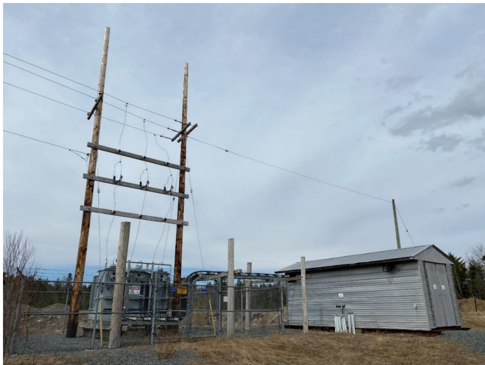
Figure 18-5: Mine Dewatering Transformer and Substation
