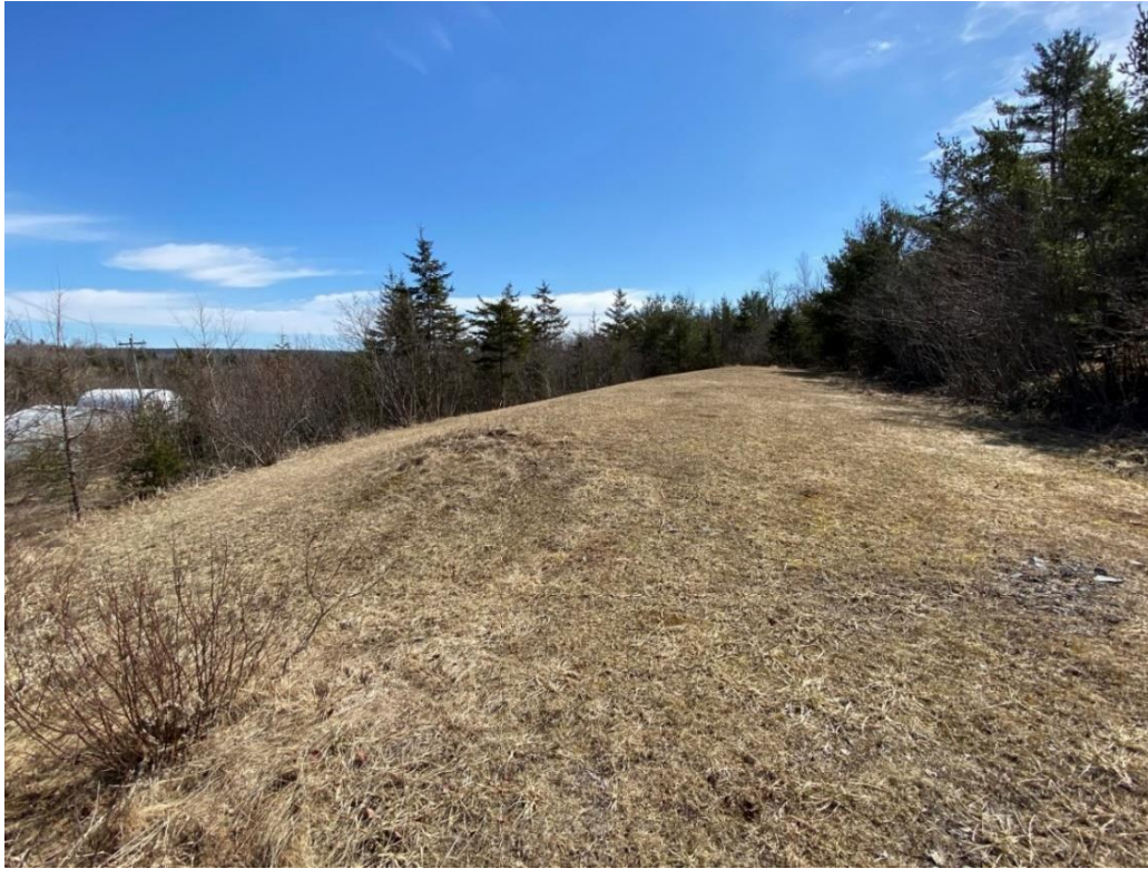
Figure 18-52: Effluent Treatment System – Septic Leach Field
