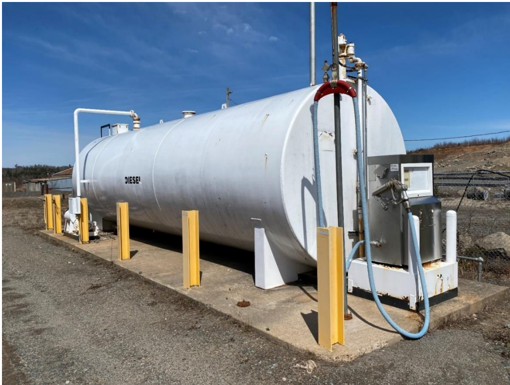
Figure 18-50: Diesel Fuel Farm
