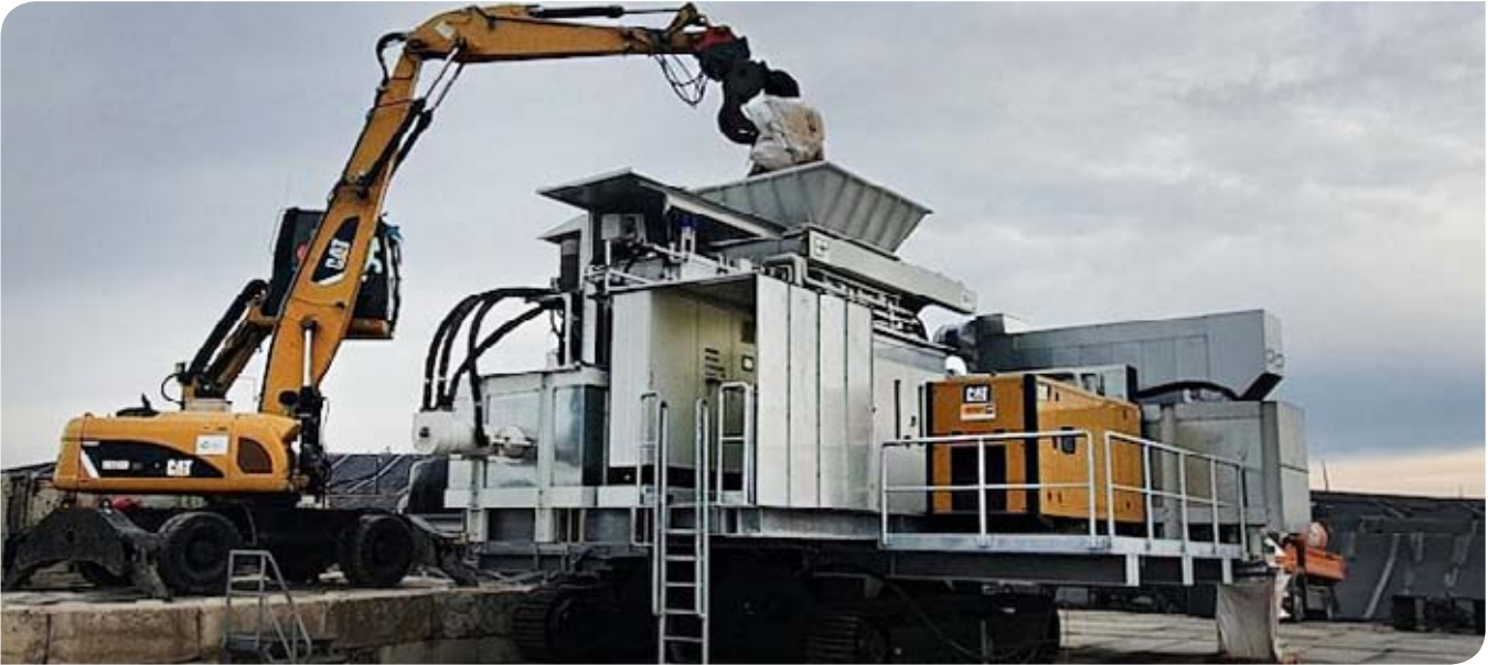
Above: Waste mineral wool is fed from above.
